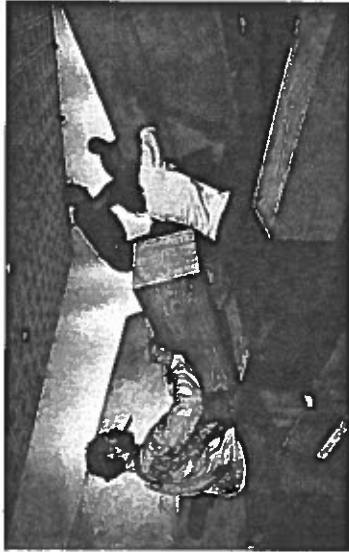
FIGURE 30 Robert Morris and workers assemble Untitled [Concrete, Timbers, Steel] , 1970. Photograph © Gianfranco Gorgoni/Contact Press Images.
